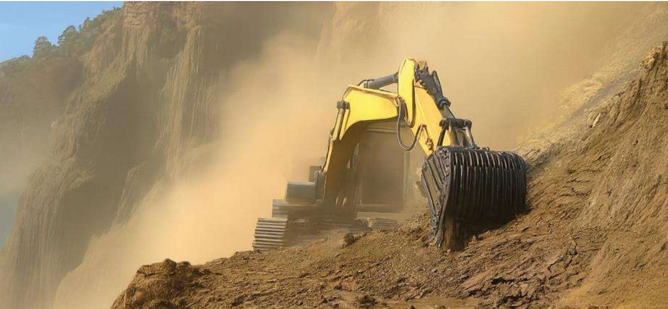
Hazardous Zone Operations
